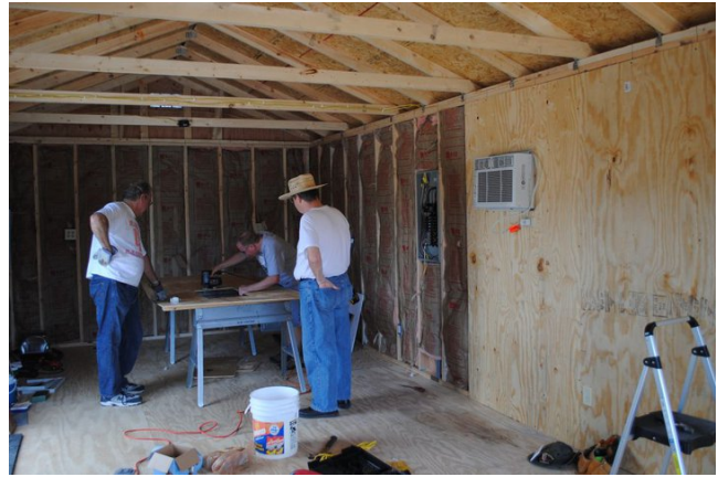
Bob Lightner, Mike Toomey and Tandy Carter putting up the insulation and walls
